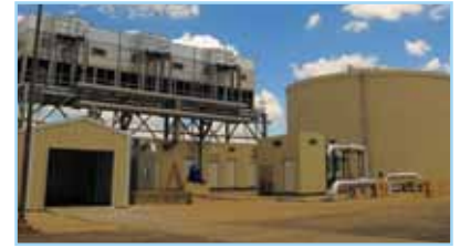
Power Plants Cleburne, TX ▶ 1.74 MG TES Tank
